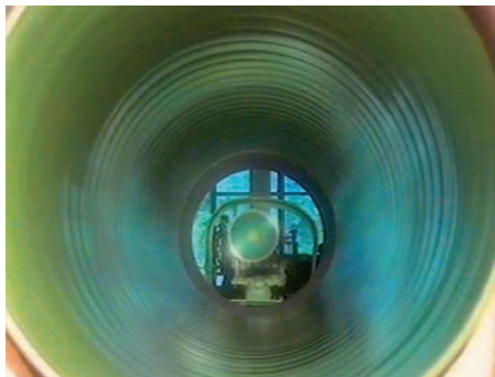
Automatic polyurethane (PUR) internal coating.
